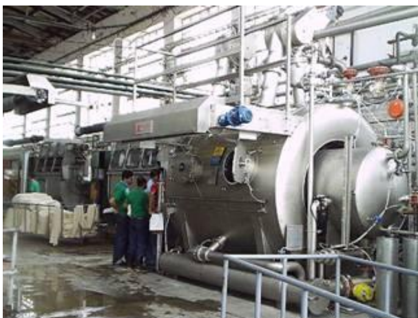
New instalations of low consumption.
