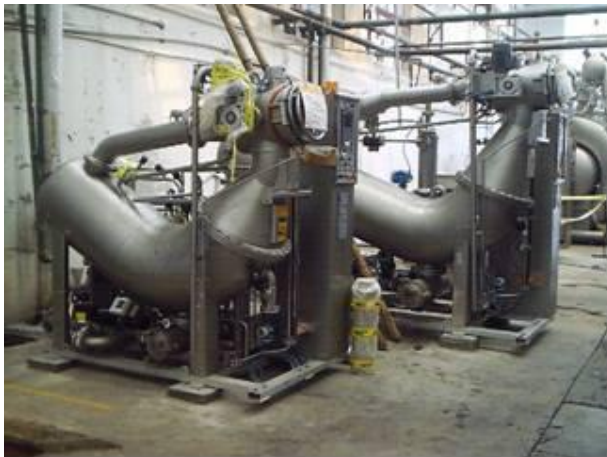
Old installations based on chemical treatment of steel
